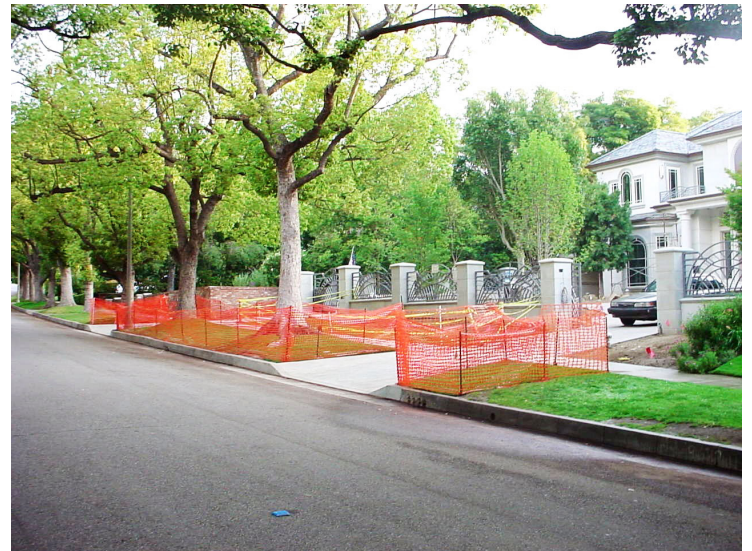
Maintain the tree protection zone fencing and parkway condition at all times.
